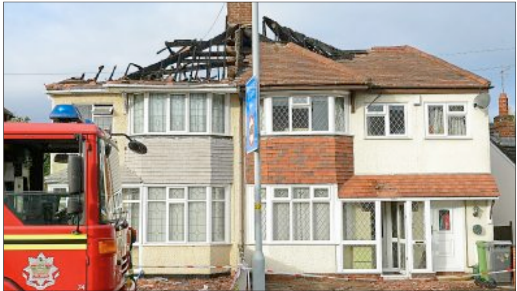
Much of the roof was destroyed while a neighbouring house also suffered serious damage
